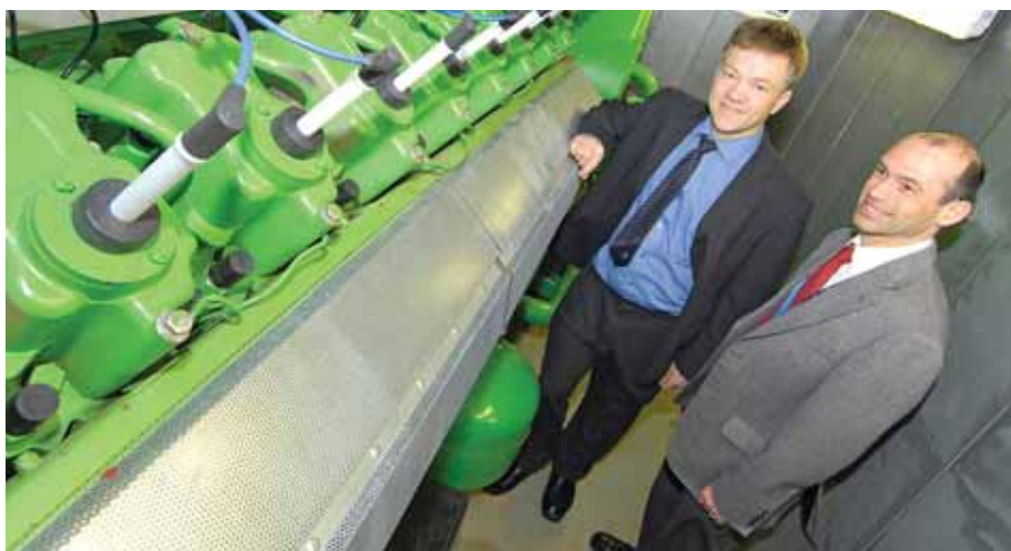
The University of Southampton won a prestigious Green Gown Award this year for its combined heat and power system. The £3 million system reduces the university's carbon emissions by over 2,000 tonnes of CO 2 a year. Pictured is one of the generators with Southampton's Energy and Design Engineer Mark Turner (left) and Neil Smith, the university's Environment Manager. The Green Gown Awards are part of the Higher Education Environmental Performance Improvement project and recognise innovative sustainable action by universities and colleges across the UK.
